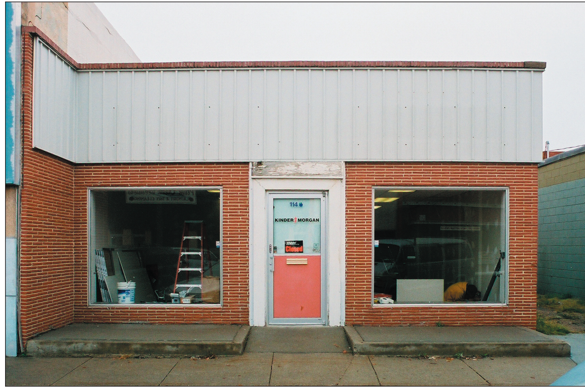
Image 1: Existing condition. Ribbed metal siding covers the top portion of the front facade. The glass front door has been modified with a metal panel and mail drop slot on the lower half.
