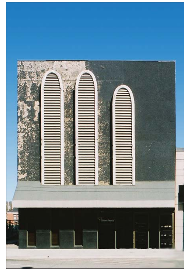
Image 3. Existing Condition. In more recent years, the second story was vertically divided to encompass a third story in the building. The building façade was dramatically altered by the addition of a false front, consisting of butt-joined plywood sheets with stone aggregate applied to the surface. Now deteriorating badly, this false front covers the entire second and third stories of the building and includes three arched elements, constructed with wood frames and louvers that cover the second and third story windows.
