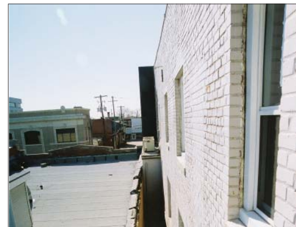
Image 6. Front Façade Wing Wall. This view from the building's rear fire escape, looking west, shows the back side of the wing wall projection of the building's west front façade above the enclosed stairway leading to the second story.
