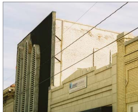
Image 5. Front Façade Wing Wall. The wing wall above the enclosed stairway on the south side of the building, viewed here from the southwest, is stabilized with braces attached to the south wall of the building.
