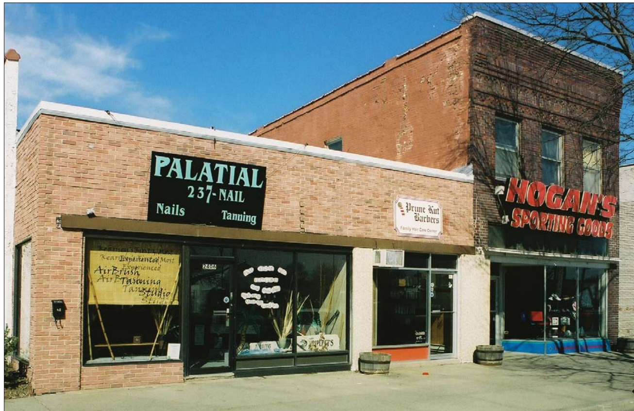
Image 2. Existing Condition: The façade of the one-story portion of the Helleberg Building currently is covered with Z-Brick or some other brand of imitation brick facing. A variety of other surface materials have been applied to the building over the years, and discordant signage now further compromises the original architectural integrity of the façade.
