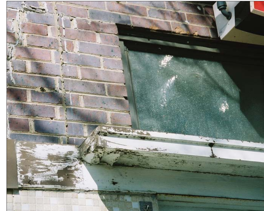
Image 4. Existing Condition: The original transom windows, with textured glass and original metal storefront window frames, still exists on the two-story portion of the building. Presumably, the same type of transom window still exists beneath the Z-Brick or some other brand of imitation brick facing that was installed on the one-story portion of the building. Underneath the transom window is a protruding lip, below which an original retractable awning presumably was mounted.
