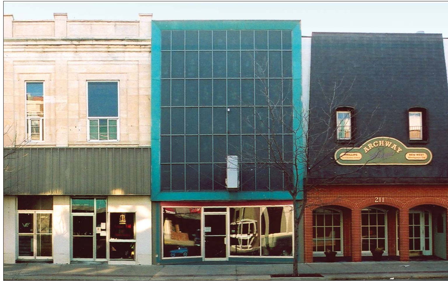
Image 3: Existing Condition. In the mid-1960s, a substantial plywood and metal false front was installed over the upper portion of the building facade. Portions of the lower facade were covered with one-inch-square ceramic tiles. Because the false front remains entirely intact, the condition of the original facade is unknown. The large second story windows are still in place and appear, from inspection after removal of an interior wall on the second floor, to be in fair condition. The original leaded glass transom window at the first floor storefront and the building's terra-cotta cornice have been removed.
