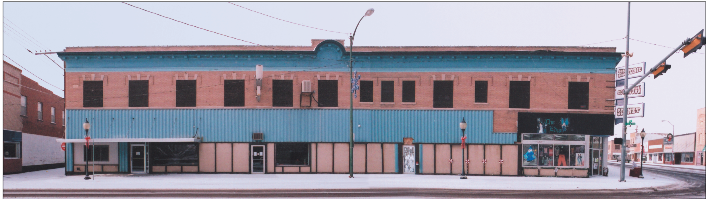
Image 2. The existing condition of the east 10th Avenue elevation of the Cleburne-Gaston Building shows that the original facade has been severely compromised by alterations, including the application of corrugated and textured panels to a large part of the facade.
