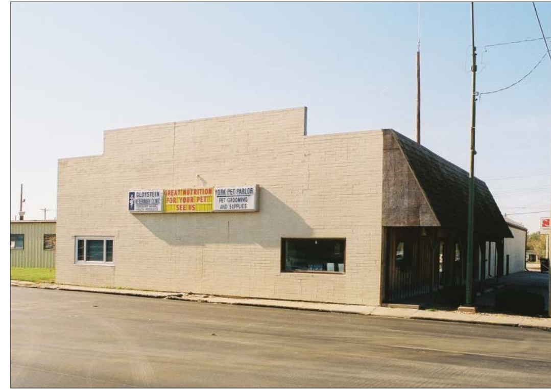
Image 2. Existing Condition. The building's customer entrance on the north façade is visible in this view from the northeast. The entrance is now situated under a large wood-framed canopy with a steeply-sloped, wood-shingled, front surface.
