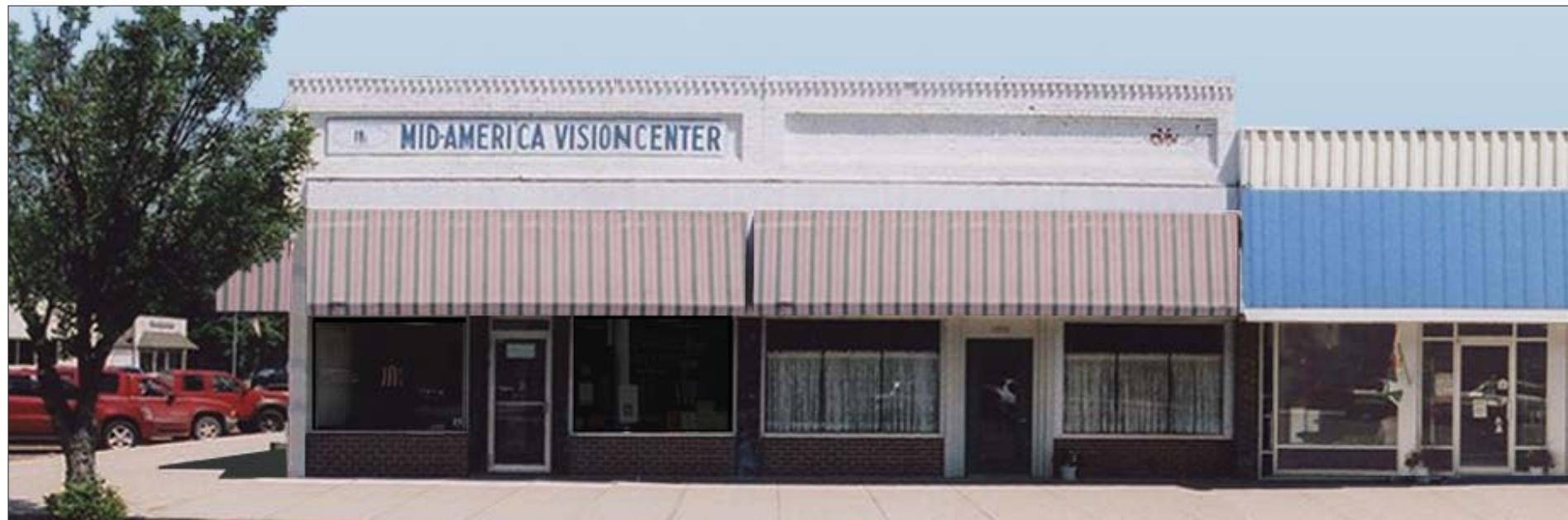
Image 2. Existing Condition (South Façade): The bulkheads below the storefront windows are unpainted red brick. In an earlier remodeling of the building, a bulkhead was built above the storefront windows across the entire south façade. The existing awnings are mounted on this bulkhead. The building's original, intricately detailed, cast iron columns remain exposed at the corner and on the Mid-America Vision Center portion of the front façade.
