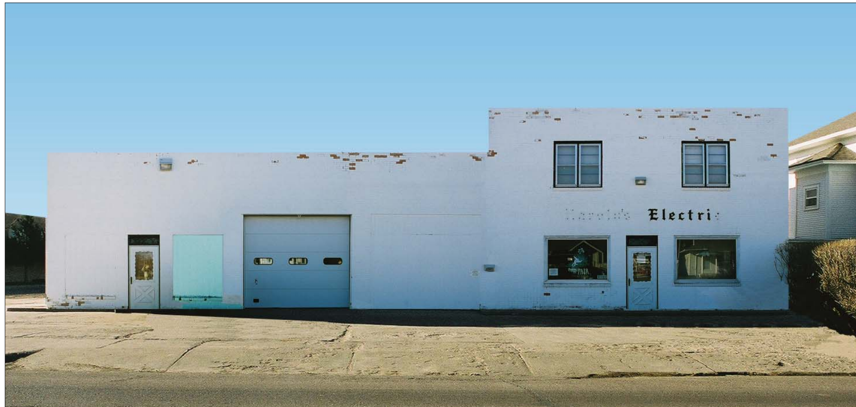
Image 2. Existing Condition (North Facade): Peeling paint and spalling brick can be seen at the roof level and near the ground on the north facade. The building's signage is also in a state of disrepair.
