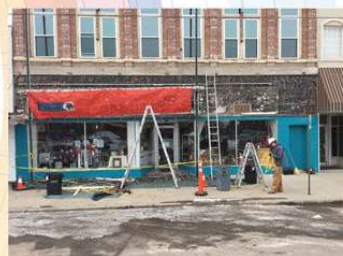
Above: Construction is underway at Mr. Dukes Mercantile. At left: A panoramic photo creates the optical illusion of a curve where isn't one on the brand-new store front that welcomes customers to Gene's Barber Shop and York County Title Co.
